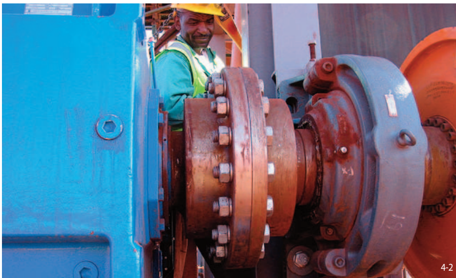
Tru-Line Flange-Coupling RFK 350 F - 350 M connects the gear of the drive unit to the head drum of an iron ore conveyor belt system in South Africa
